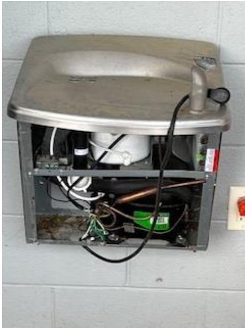
Fixed water fountain at the swimming pool.
